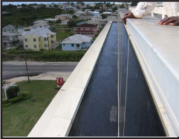
GUTTER ON EDGE OF BUILDING NOT SUITABLE FOR SPRAYING
